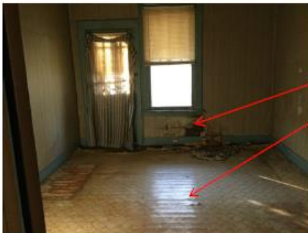
Interior wall damage due to window Floor covering in disrepair
