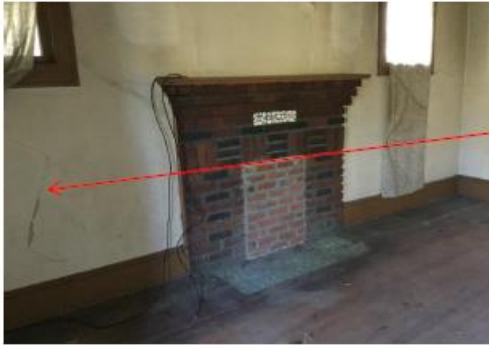
Interior walls have cracks
