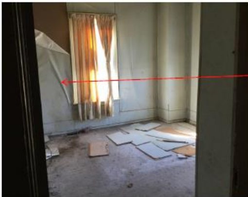
Interior walls in disrepair
