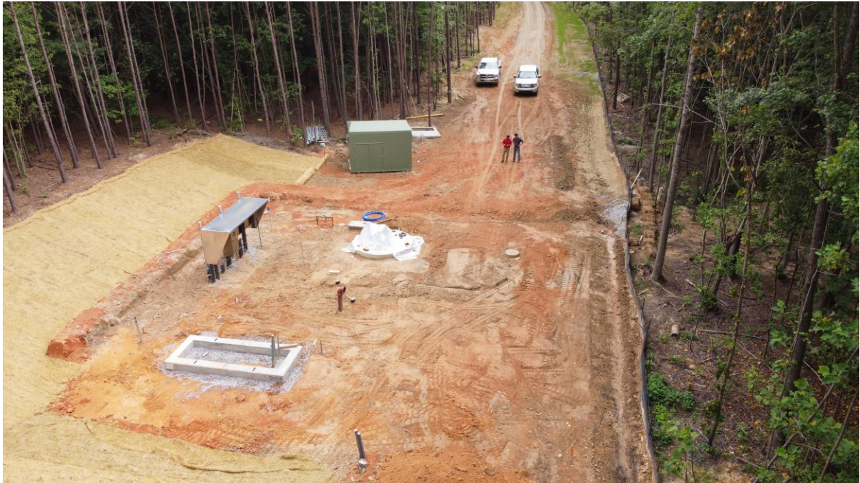
Pump station site coming along with the erosion control measures in place.
