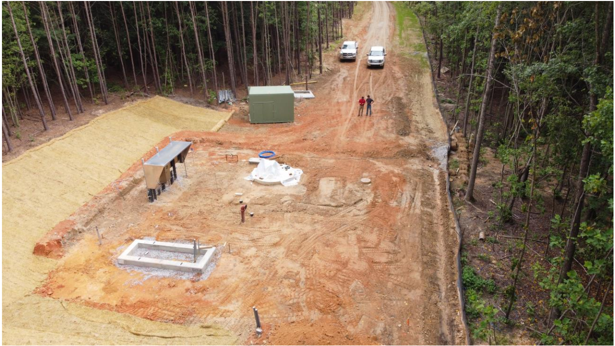
Pump station site coming along with the erosion control measures in place.
